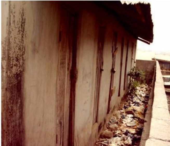
Figure 2. The rear side of the public toilet being used as a refuse dump.
